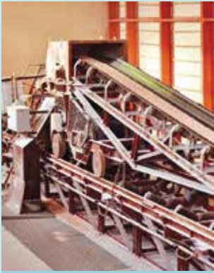
Travelling tripper for efficient and automated material distribution.
