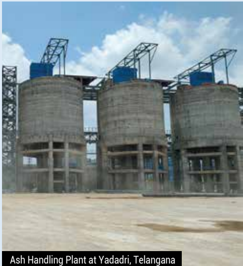
Ash Handling Plant at Yadadri, Telangana
