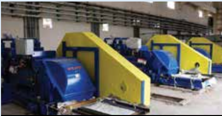
High Concentration Slurry Disposal Pump at Yadadri
