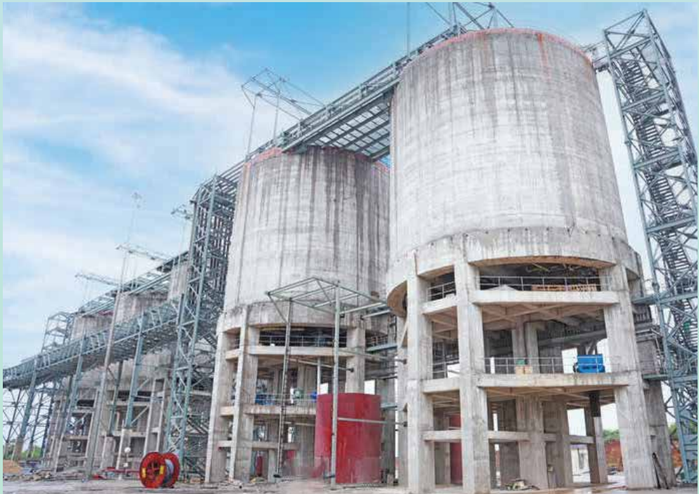
Ash handling plant at Yadadri, Telangana
