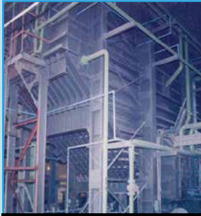
Bottom Ash Hopper Arrangement
