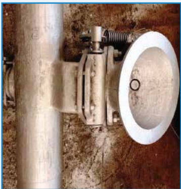
FLY ASH INTAKE VALVE
